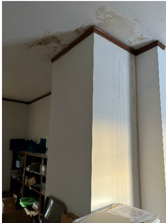
Photo 10 – Water damage at chimney penetration through roof
