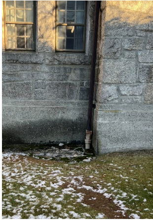
Photo 7 – Water staining below damaged gutter
