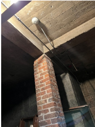
Photo 1 – Brick pier, concrete and masonry wall beyond, concrete beam and flat slab
